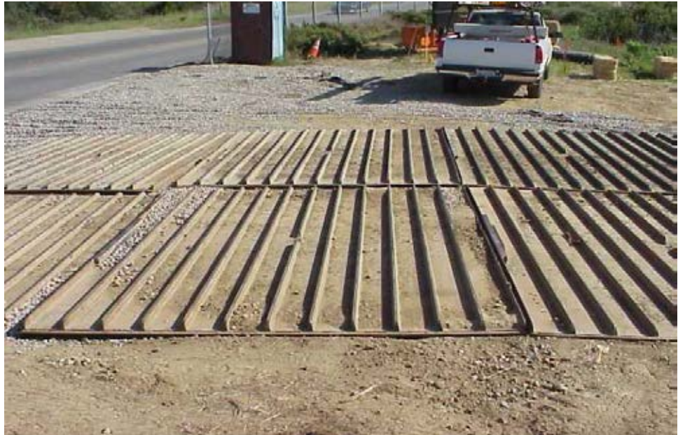
Manufactured metal plates knock dirt off vehicle tires before exiting a site.
